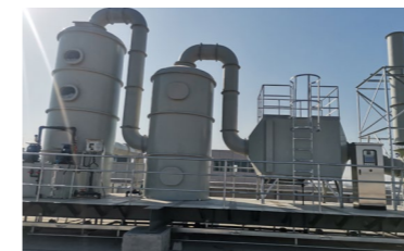
Class C hazardous waste storage waste gas treatment facilities
