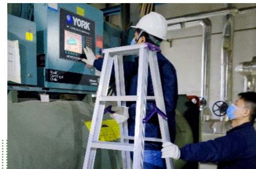
Optimizing air conditioning operation modes
