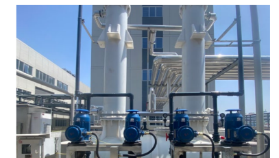
Falling film absorption tower
